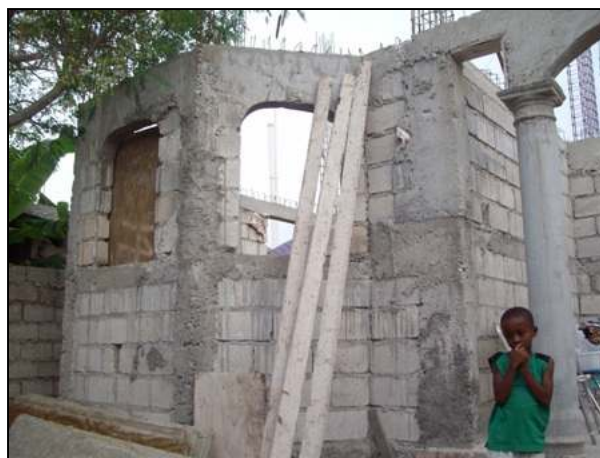
The new house, ready for a roof. As soon as the roof is up, his family will move out of the tent and into the house while construction is completed.
